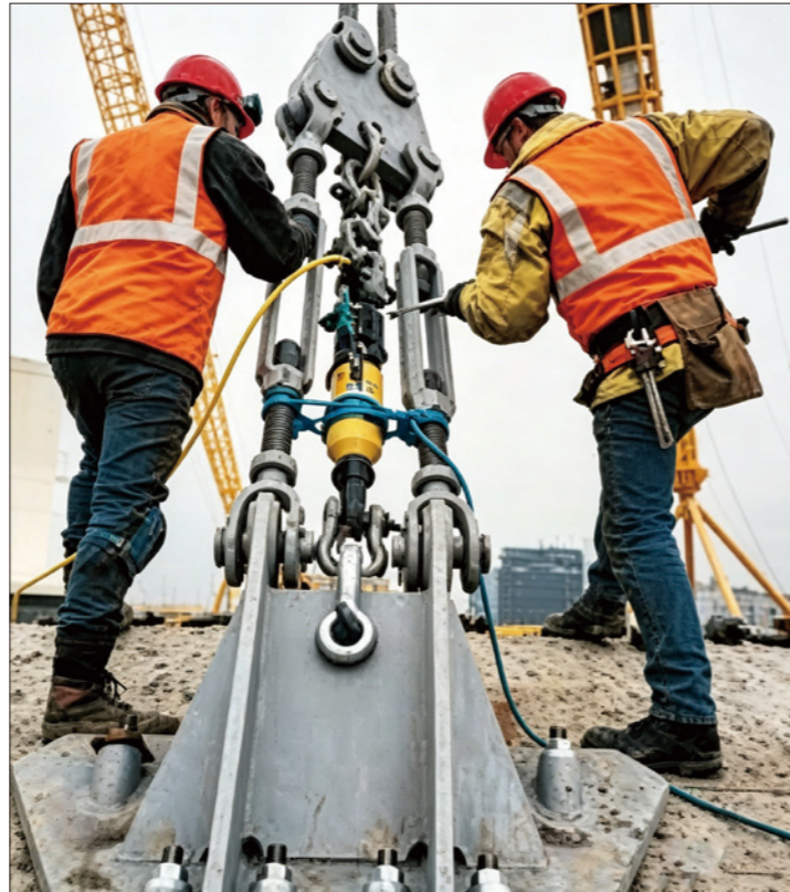
▼ To lift a load bearing mast into place, BRP-Series cylinders were used to tension the supporting cables.
